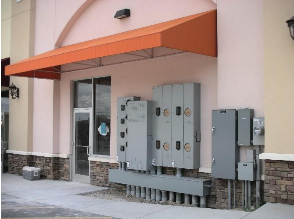
Prohibited (utilities facing street)
